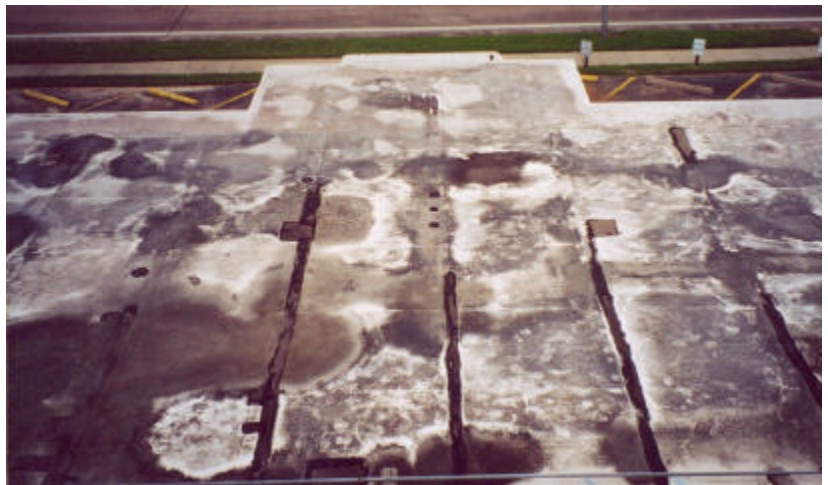
No matter how much you try to prevent it, white roofs will become discolored over time.
