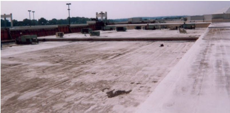
Discoloration means both seen and unseen perils to the roof's long-term performance.
