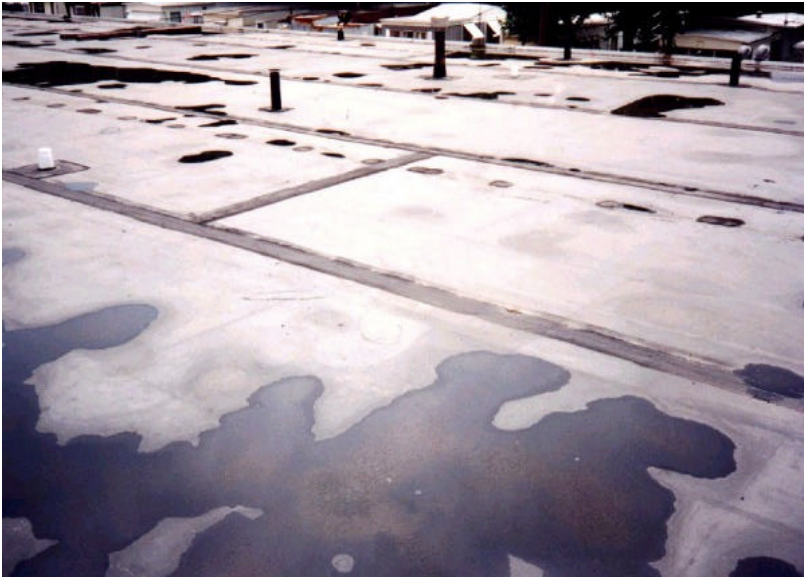
This aged EPDM roof has been repaired with newer membrane – notice the light gray reflective color of the aged membrane.
